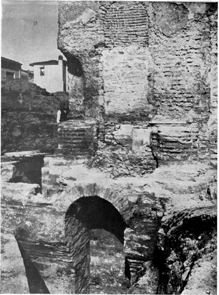
FIG. 5.— WEST END OF BODRUM CAMII, SHOWING THE LOWER AND UPPER CHURCHES. THE OUTER WALL OF THE CISTERN CAN BE SEEN TO THE LEFT, AT THE BOTTOM OF THE PICTURE.
